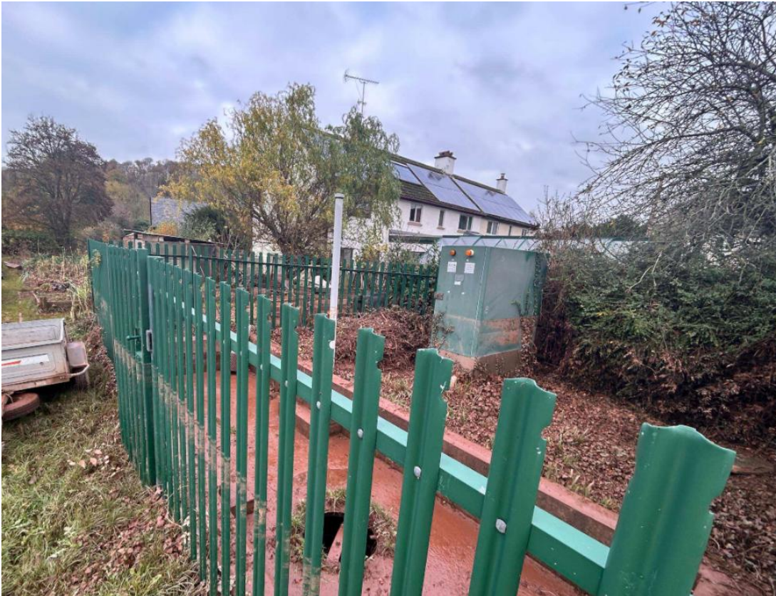
Figure 5-6 Water Level to Substation
