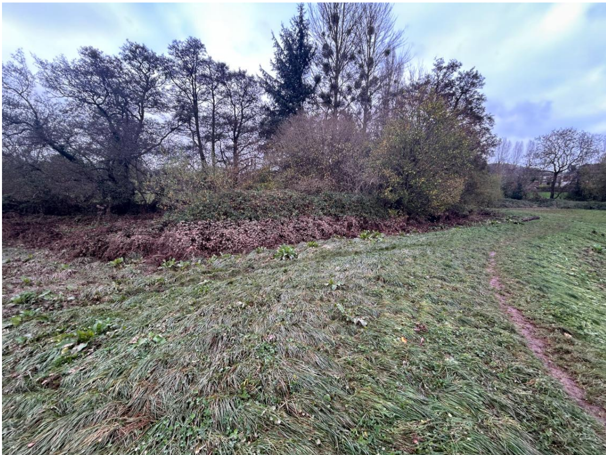
Figure 7-1 Flood Flows Across Earth Embankment Defence
