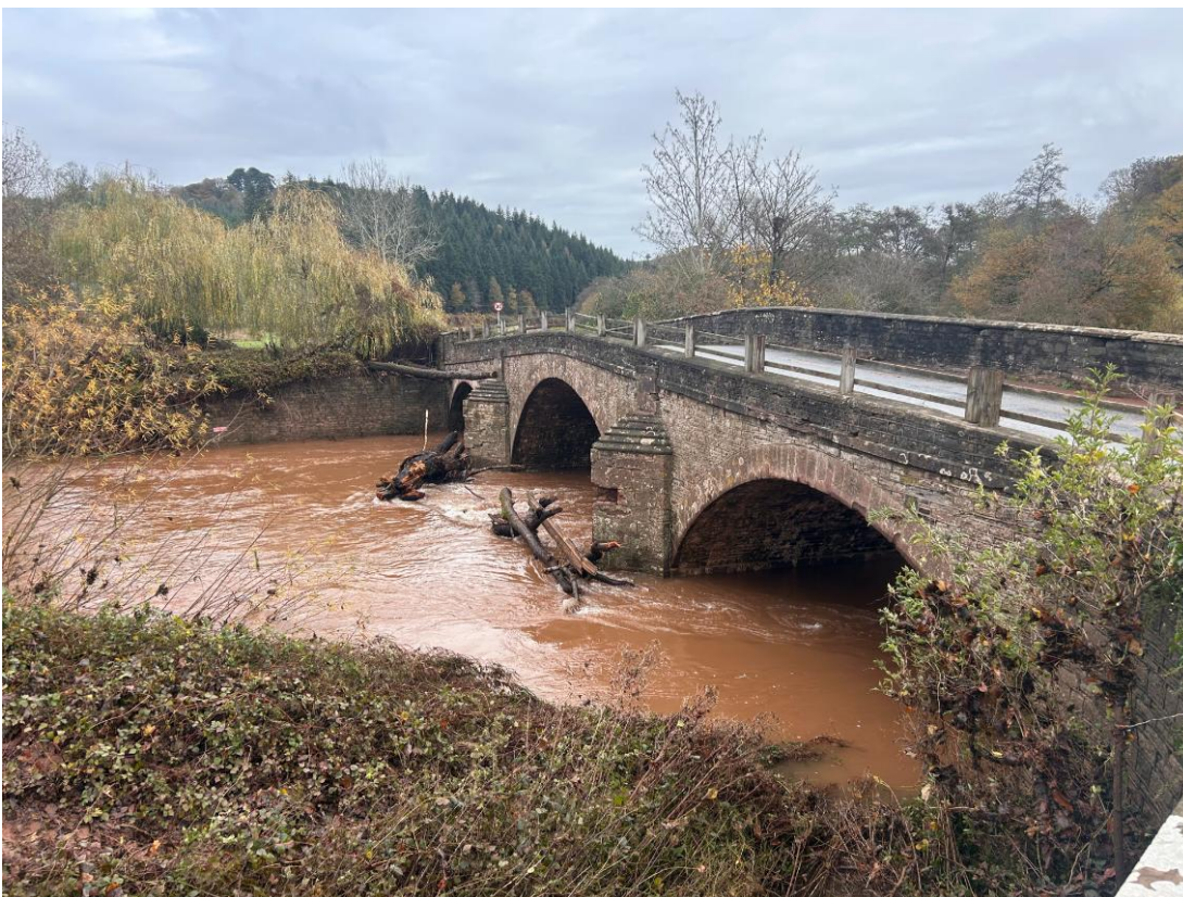
Figure 5-3 Remaining Debris on the Bridge
