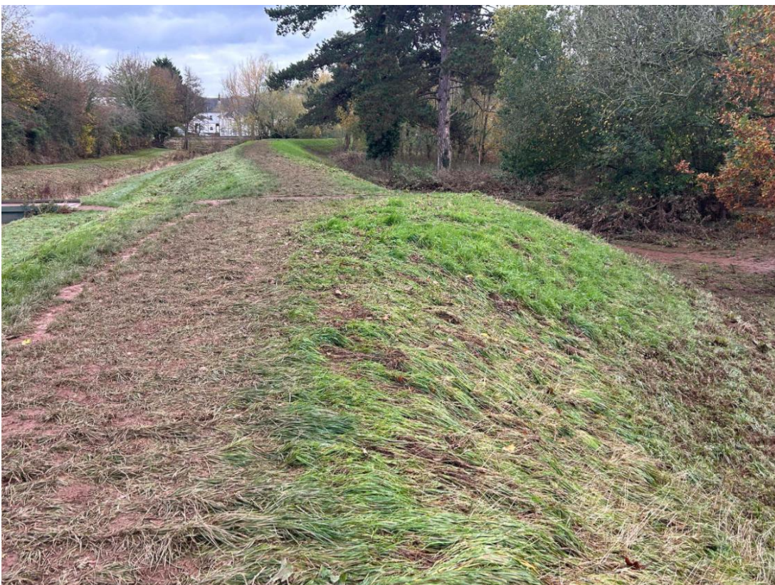
Figure 8-7 Overtopping of the NRW Maintained Earth Embankment Defence
