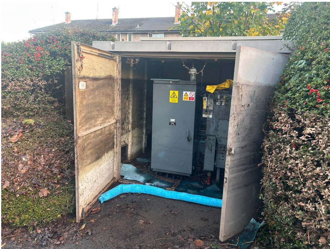
Figure 8-13 Electricity Substation on land adjacent to Goldwire Lane
