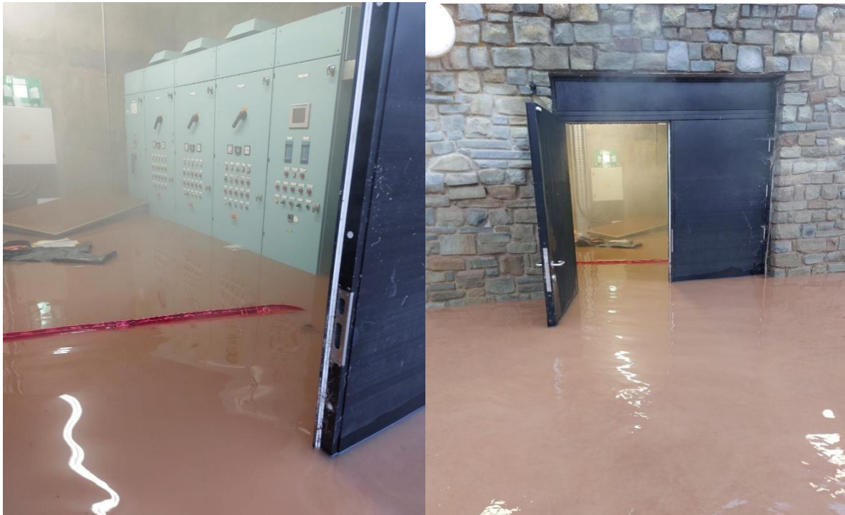
Figure 9-4 Wonastow Road Pumping Station
