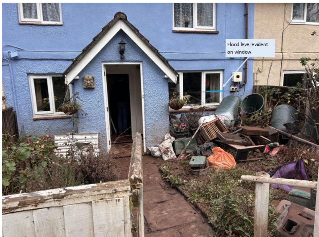
Figure 7-3 Damage to properties along Forge Road
