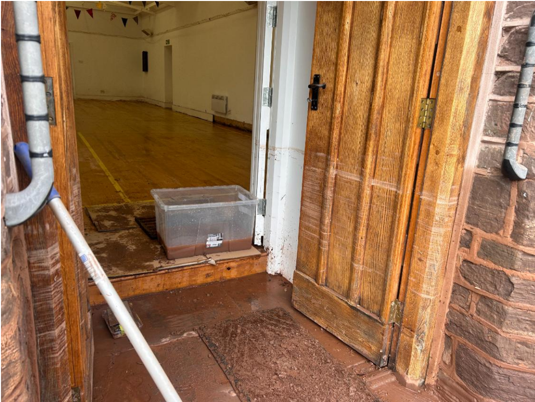
Figure 5-4 Evidence of Water Level to Village Hall
