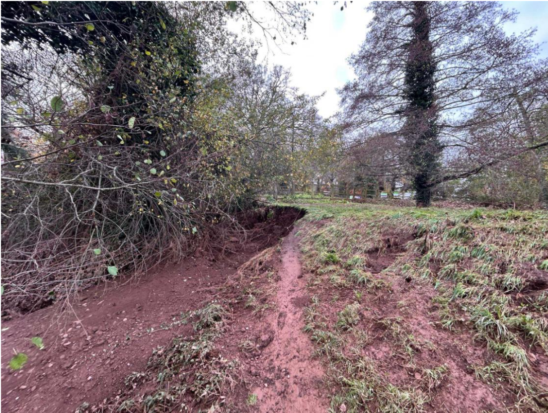
Figure 8-6 Erosion to Landward Side of NRW Maintained Earth Embankment Defence
