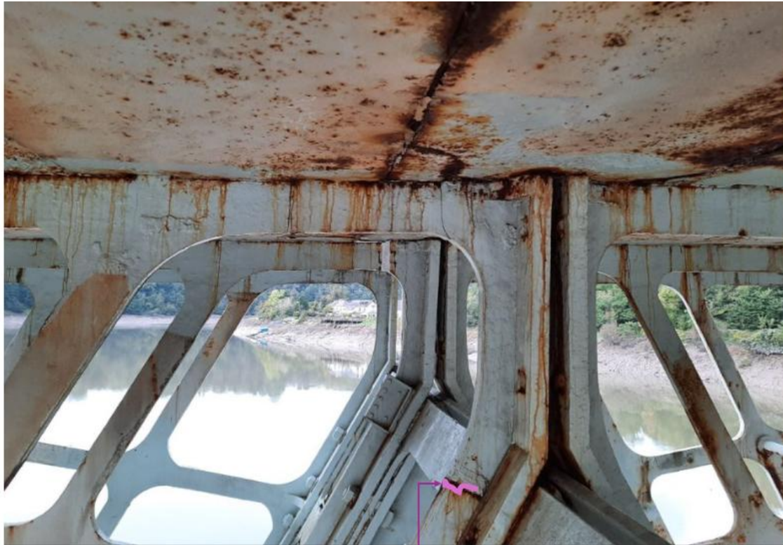
New crack location
