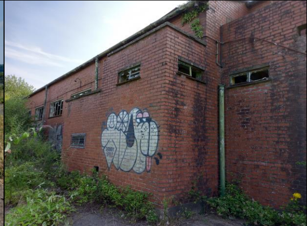
Photo EDP 2: Building B1 , an example of broken windows used for access by bats, facing north-east.
