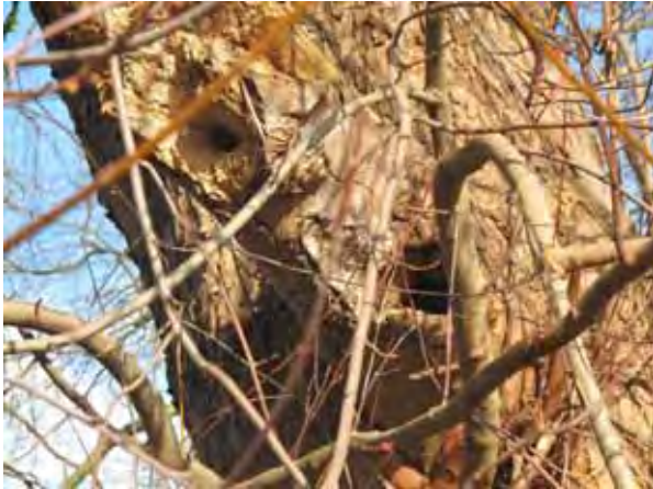
Knot holes present on eastern aspect of tree 32 (silver maple).
