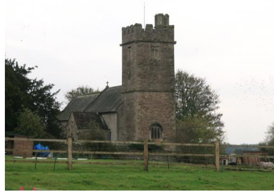
Fig.19 The Church of St Stephen and St Tathan: a mix of ashlar and coursed rubble stone with natural slate roof
