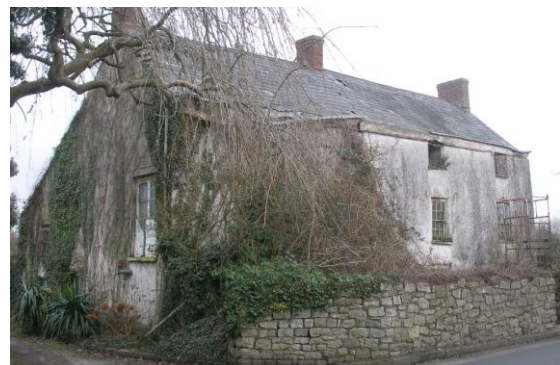
Fig.49 Caerwent House: a significant historic building in a critical state of disrepair
