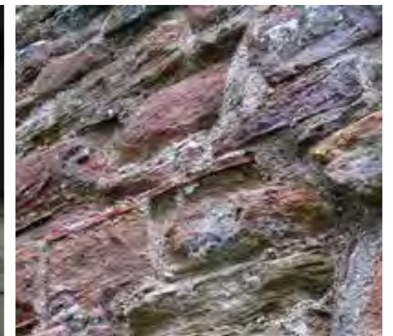
Many of the older structures are built in red sandstone. The red and buff sandstone ashlar was quarried locally and is characteristic of the area.
