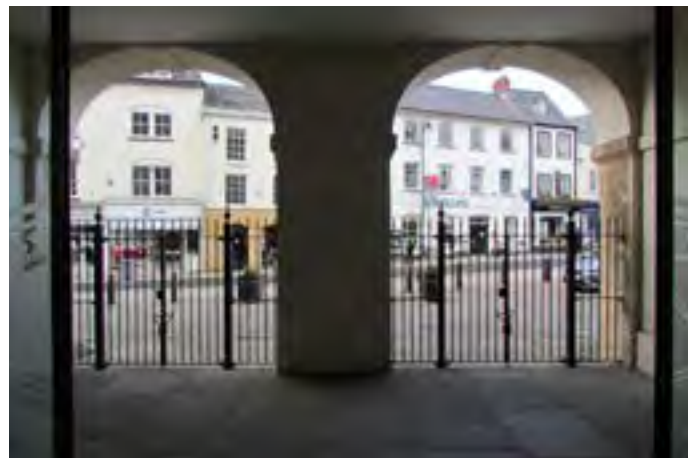
Configuration of existing railing and gates, while performing a necessary function, hinders open access to the loggia
