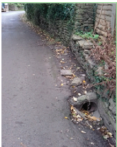
Surface water drainage inlet
