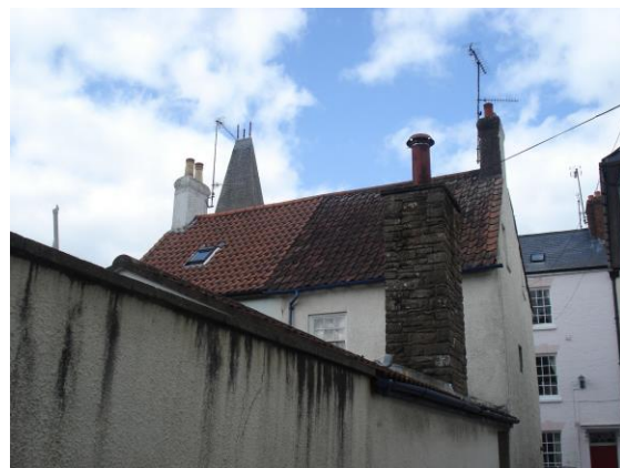
Fig.26 Pantiles are seen to roofs of more modest dwellings and outbuildings to this part of the conservation area (houses to junction of St Mary's Street and Worcester Street)
