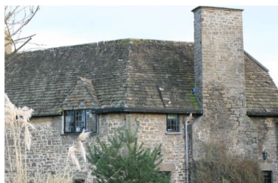
Fig.70 Sandstone is a feature of the vernacular revival houses either squared or as seen here as rubblestone
